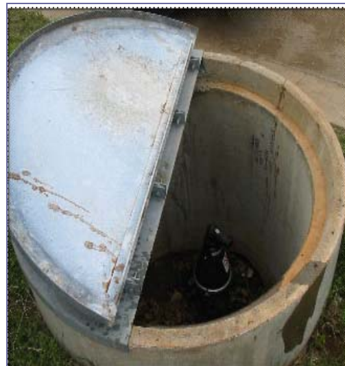
Typical Air Valve Vault D-025 Combination Sewage Air Valve
